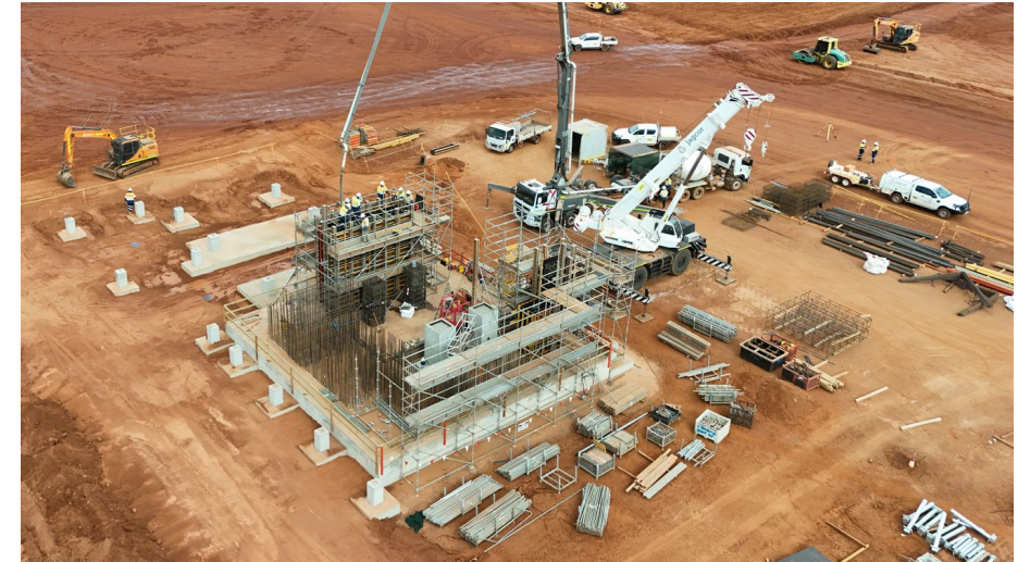
1.) Mill Slab and Feed Trunnion
