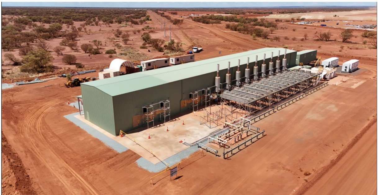
Karlawinda Expansion Project – Power station extension.
